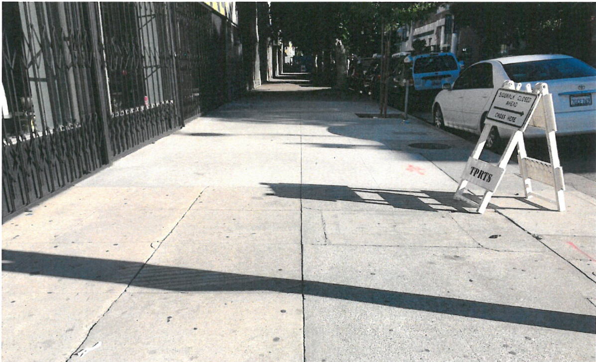
10. Condition of abutting sidewalk on Olive St., facing northeast.
