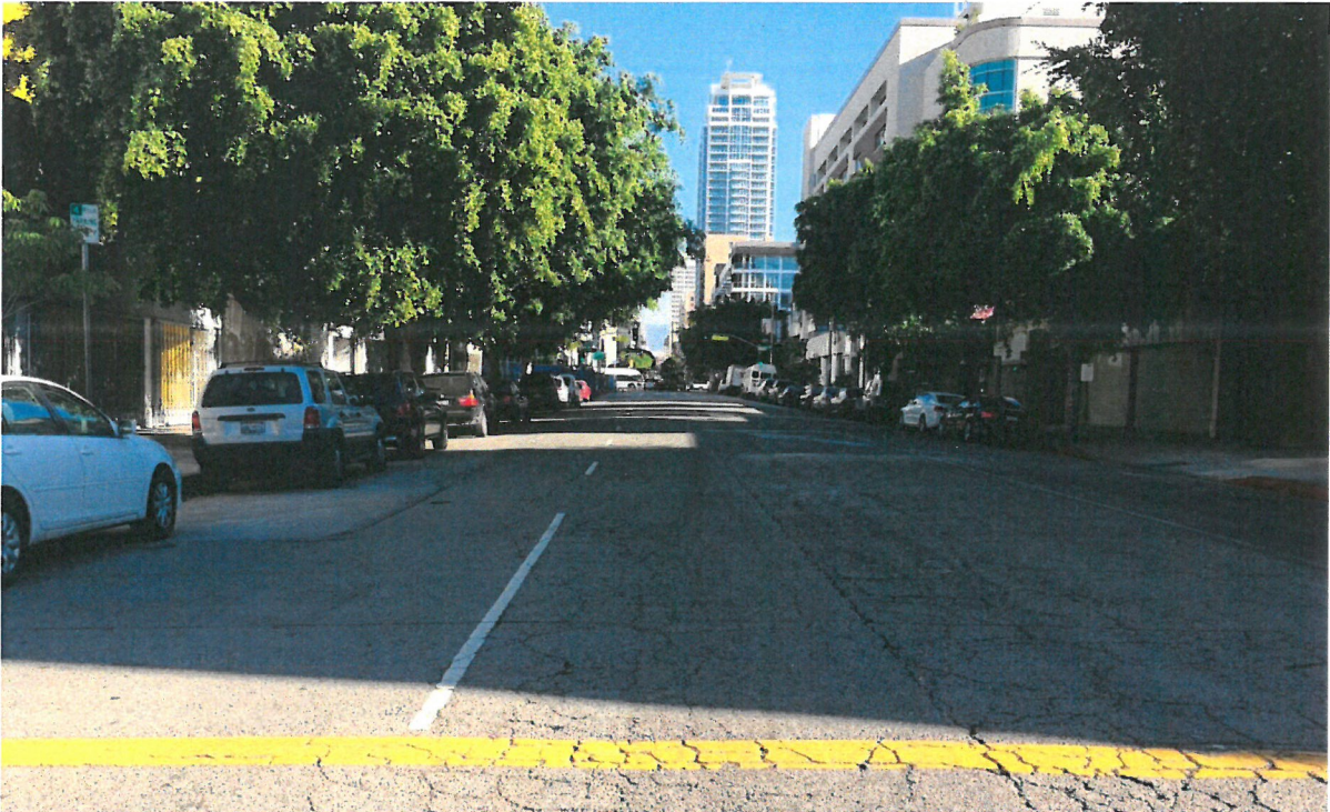
9. Condition of public right-of-way – Olive St., facing northeast.
